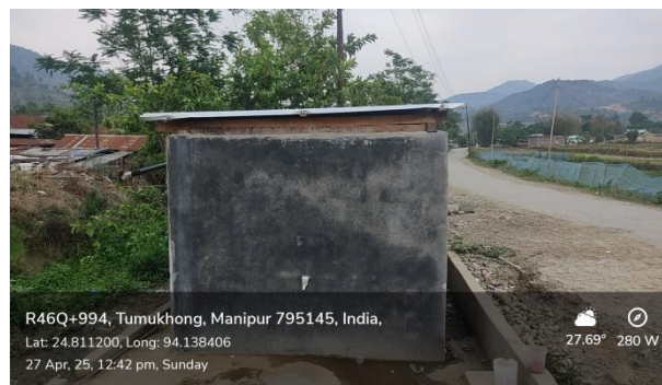
Figure 2: Water Tank at Tumukhong Village
